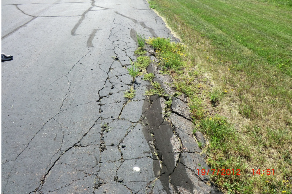
BFW RY725 001 Alligator Cracking & Swelling (PCI = 65)
